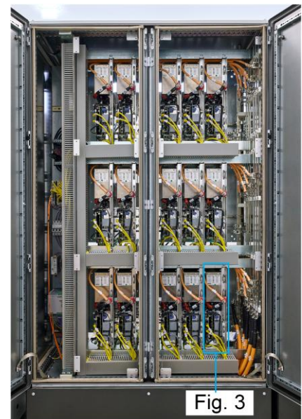
Figure 6: Insight into the load module cabinet
